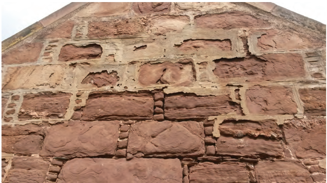
Fig. 1 (Right) The barracks at Fort George, where the damage to stonework was caused by cement mortar. The cement on this elevation was left in place by Historic Scotland to demonstrate to visitors the damage caused by cement mortar on traditional masonry.
