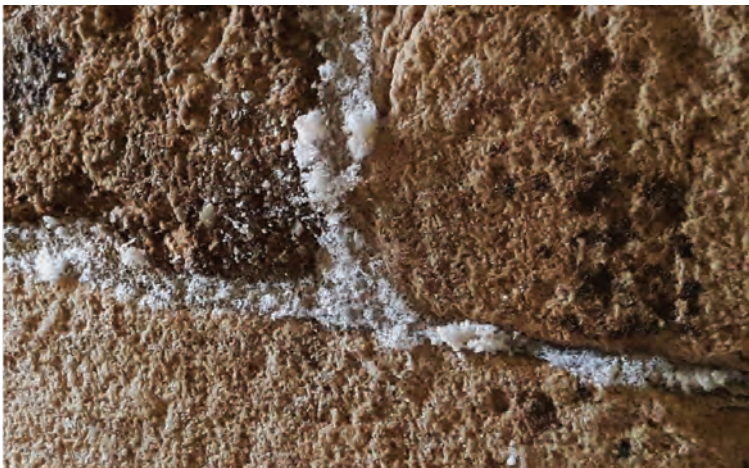
Fig. 3 (Below) A visual manifestation of traditional lime mortar's sacrificial functional behaviour at work. Underlying processes are examined in Figures 4 and 5.
