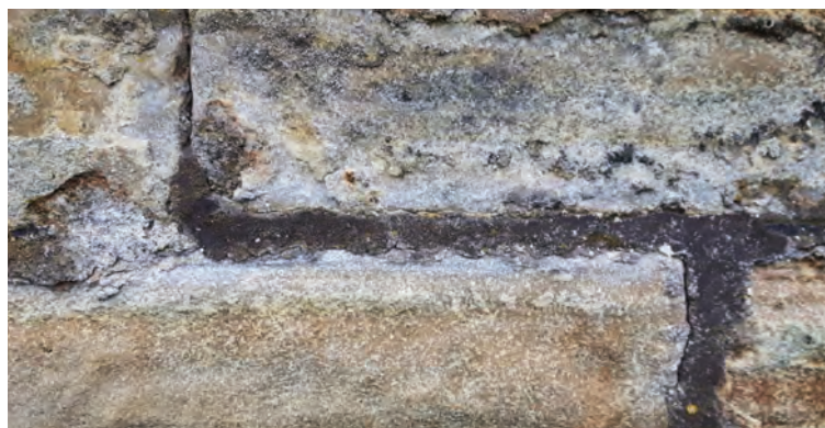
Fig. 8 (Below) A visual manifestation of the damage of cement at work: the ramifications of forcing evaporation and hence salt precipitation to occur in the arrises of the stone, displaced around the mortar joint (rather than through it, as in Figure 3).
